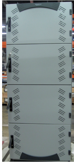
Colocation 19" enclosure Enclosure separated in 4 parts to give different access to each customer. Each hosted customer has his own secured access and cannot make some operation to the other part of the enclosure
