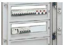
Detail from the circuit marking system.
