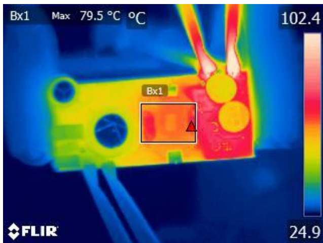
Figure 38 – Ambient = 24.9 °C. Transformer, T2 = 79.5 °C.
