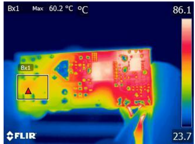
Figure 35 – Ambient = 23.7 °C. Bridge Diode, BR1 = 60.2 °C.
