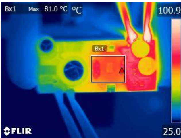
Figure 42 – Ambient = 25 °C. Transformer, T2 = 81 °C.
