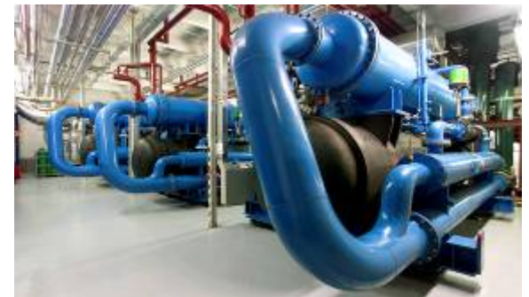
30 MW cooling capacity
