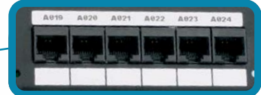
Patch Panel / Face Plate Labels
