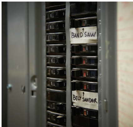
Label electrical components: 3M™ Masking Tapes ( pgs 57-60 )
