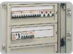
Detail from the circuit-marking system.
