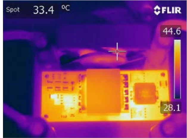
Figure 19. Thermal Image of the ADP1074 with Air Cooling Provided by Fan, 1 Hour Soaking Time
