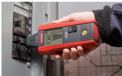
Identify the single correct breaker
