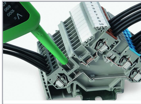
Testing via voltage tester directly on the current bar.
