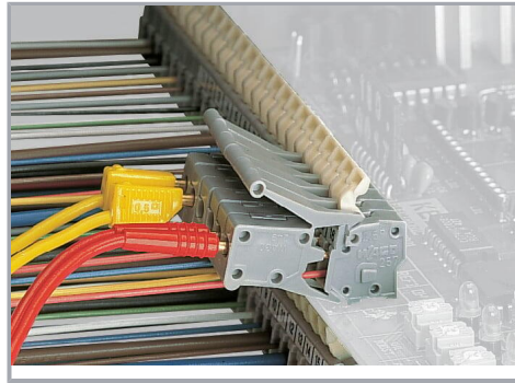
Testing with test plug modules.
