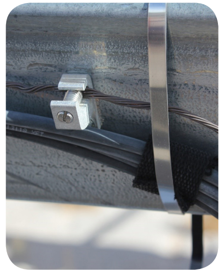
In the image above, effort was made to protect the cable jacket from potential abrasion from a metal cable tie. The risk is that this small piece of insulation may erode or slip and leave the cable jacket exposed to the metal tie at an unfortunate angle.
