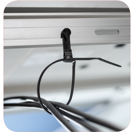
The nylon cable tie looped through the module hole is unlikely to last more than a year or two on a single-axis tracker application.
