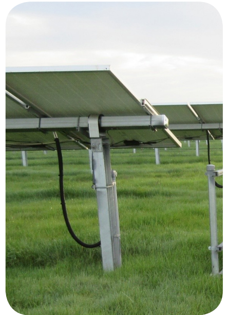
The tubing used on the wiring in this photo would seem to protect the wires from damage. The long, loose run actually encourages damage from lawn mowing equipment and the wind.
